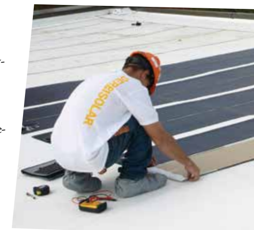
A Cornell Roofing & Sheet Metal employee installs solar panels on Bayer CropScience's roof system.
